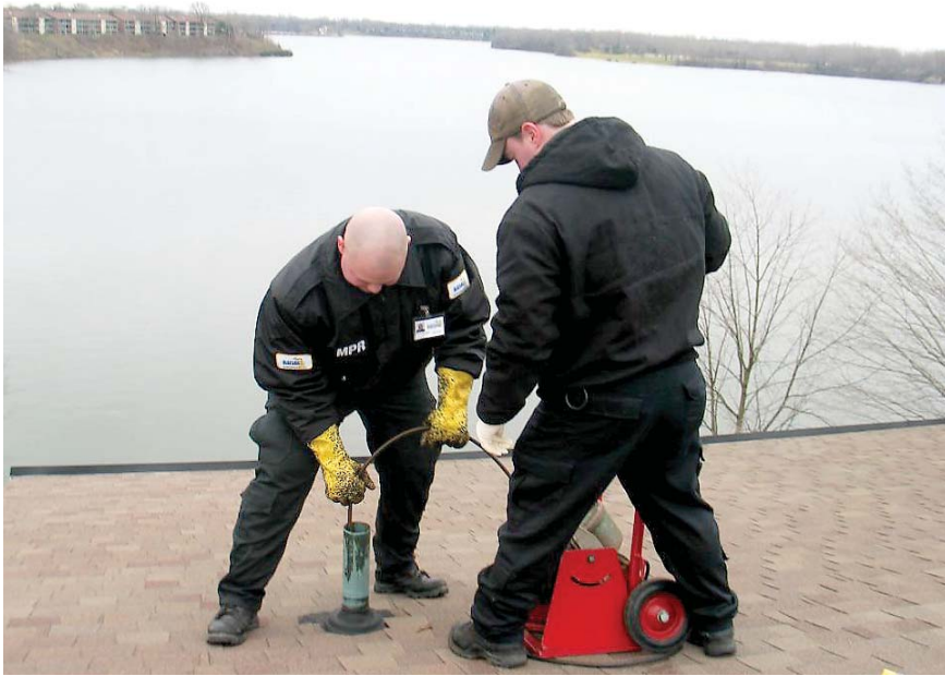
Technicians Tom Rieder (left) and Adam Carman clean debris and sludge from a roof vent atop a 2 1/2-story condominium.
